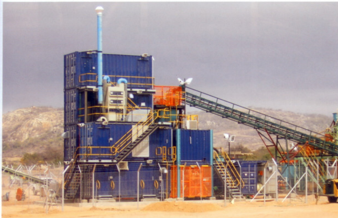
A containerised Ultrasort recovery unit at the Murowa diamond mine near Zvishavane in Zimbabwe. Supplied by ADP, it is capable of treating 1 t/h of -16 mm DMS concentrate material.
