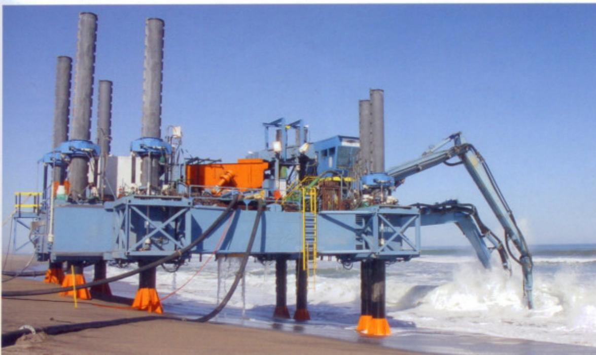
An ADP 'jack-up platform' mining system working in the surf zone for Namdeb on the southern coast of Namibia.
