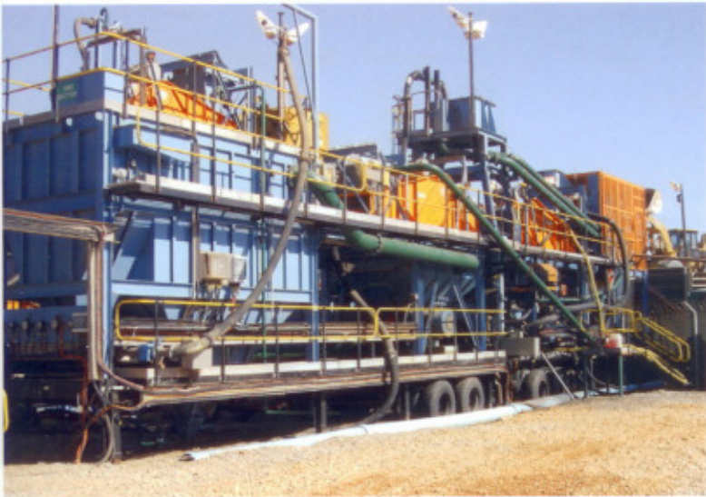
An ADP process plant at one of Namdeb's 'Pocket Beach' operations in Namibia.
